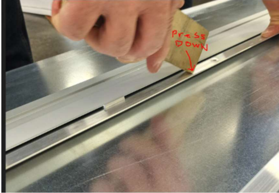
Figure 7: Use hand tool to apply pressure. Pass over entire hanger bar 4 times.
