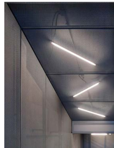
MESH CEILINGS WITH HIDDEN LINEAR LIGHTS
