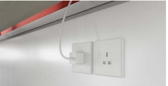
Sophisticated Power Solution Diversal's robust power and data system is seamlessly integrated for easy access and maintenance. Dual cable way allows segregation of power and data cables.
